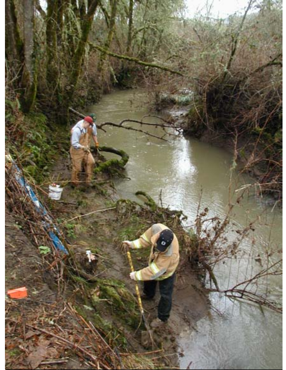
Greg McDowell, Brian Kohlmeyer, and Cody Rich of the Perrydale FFA plant willow cuttings along Muddy Creek to help stabilize the banks.
